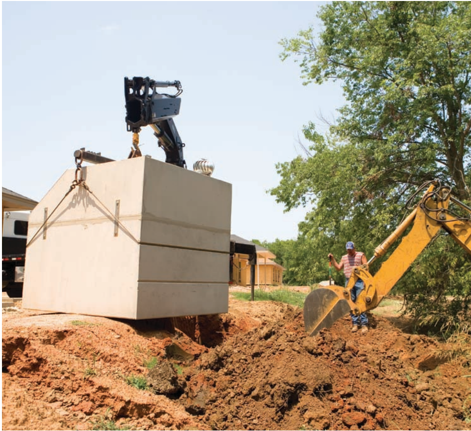
A crew installs one of 125 storm shelters provided to Chickasaws in 2006 through the tribe's housing division.
