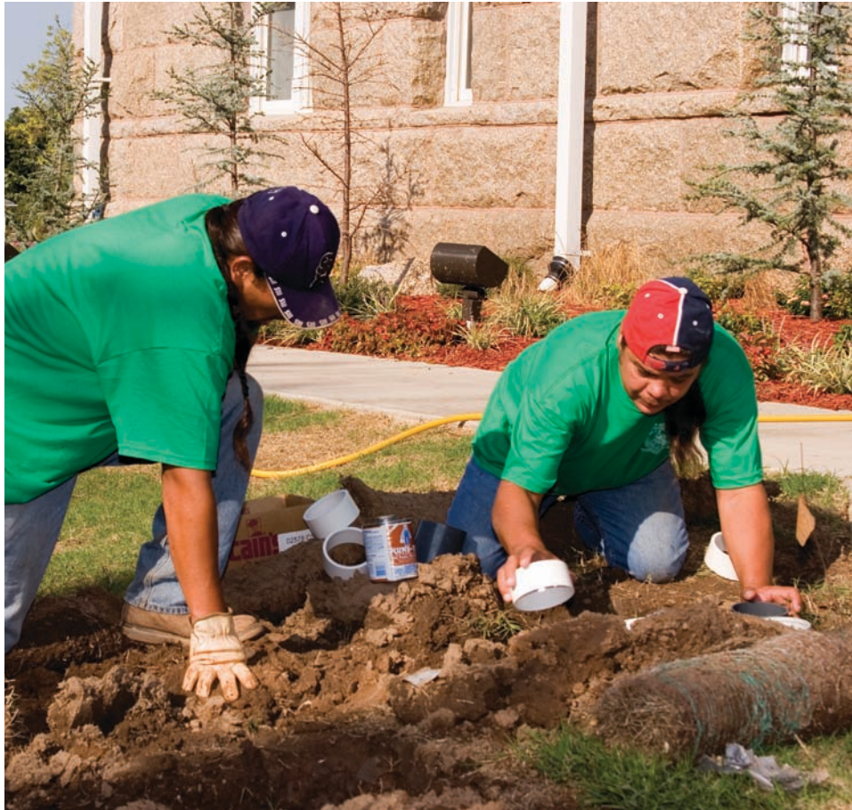
Jay Wisdom and Michael Markum work together installing a lawn drainage system at the Chickasaw Capitol grounds in Tishomingo.
